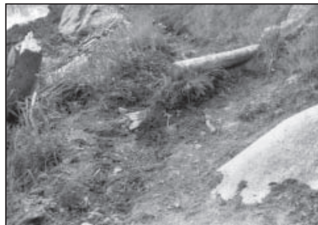
Figure 4—Too much water and sediment washed this waterbar out. Keep the water moving until you get the suspended soil where you want it. This sounds simple, but most failed water diversion structures are ones clogged with deposited soil.
